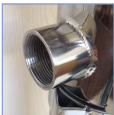
Fittings and walls: stainless steel 6 mm
